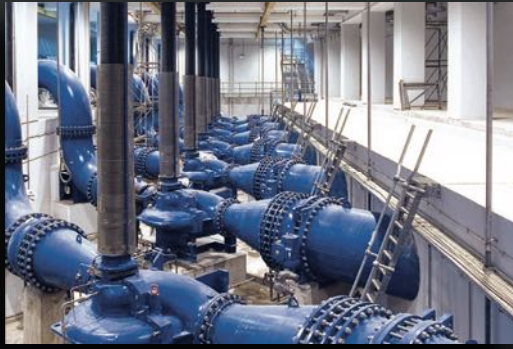
Pumps and compressors
