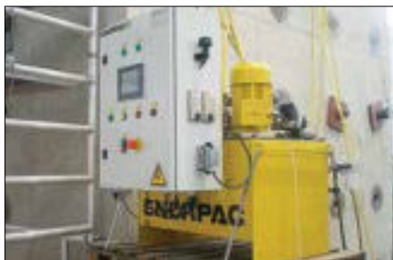
◀ Custom pumps with control packages.
