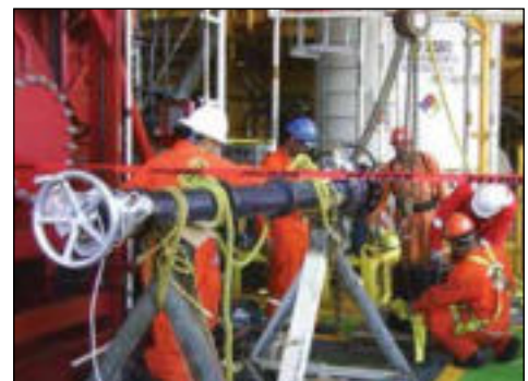
▼ CHT2000 hot tapping offshore application.
