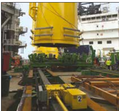
▼ The trolley system speeds up offshore wind transition piece load out: the transition pieces are positioned in the clamping frames and moved along the track.
